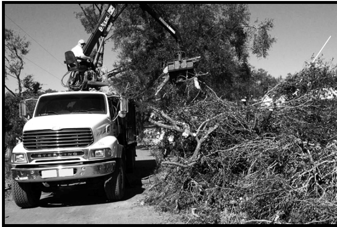
Figure 3.1 - Typical Vegetative Debris on a Public Right-of-Way
