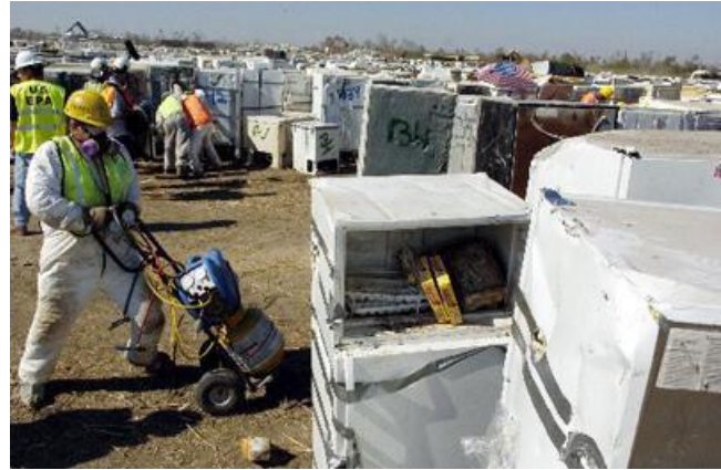
A licensed technician removing Freon from refrigerators at a TDMS waterway debris in Livingston Parish, LA. Ceres has also completed waterway debris removal in Iowa, Georgia, South Carolina and Florida.
